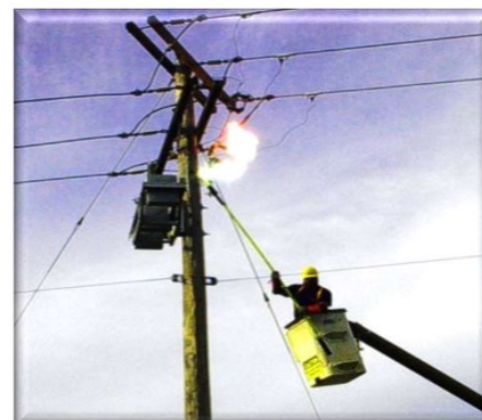
Figure 43 Example of why a load buster on a stick should be used on capacitor banks.
