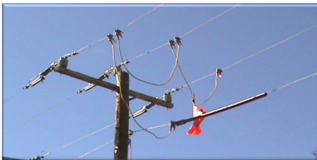
Figure 28 Short Circuited, Grounded & Flagged
