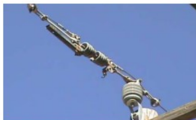
Figure 22 De-energized Visible Opening
