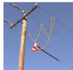
Figure 25 Flagged, Tagged & Grounded
