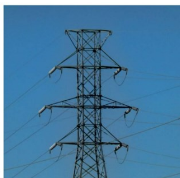
Figure 47 Lattice Tower Angle Structure With Horizontal Insulators
