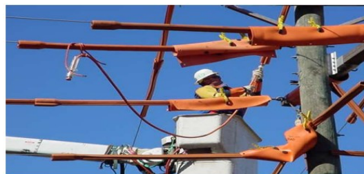
Jumper end secured with collar rope
